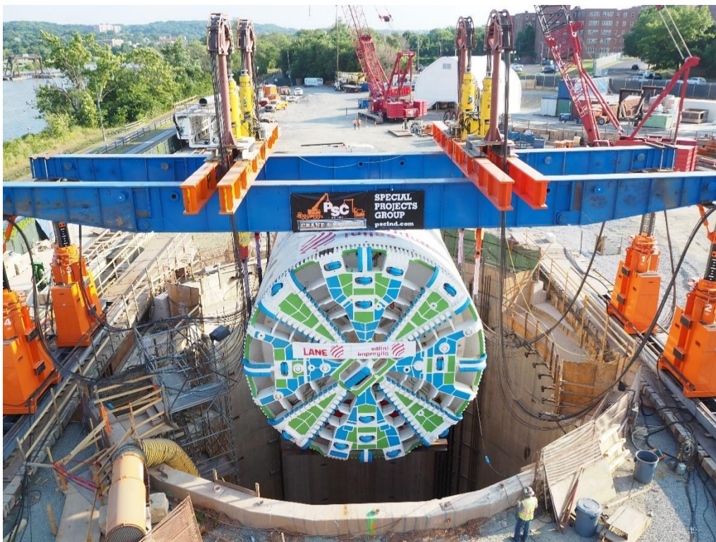
Figure 8. Example of a Large-diameter TBM Cutterhead and Shield Being Lowered into a Main Work Shaft
