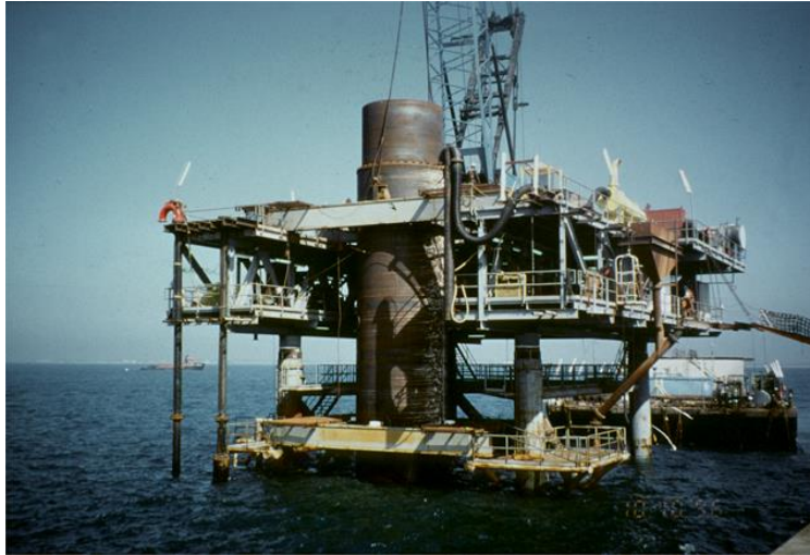
Figure 7. Example of a Vertical Conveyance Shaft Being Lowered Toward a Tunnel at Sea
